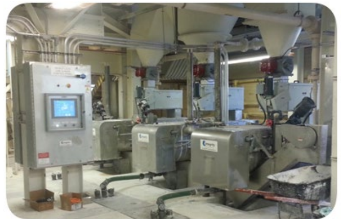
Davis WTP, Austin TX
