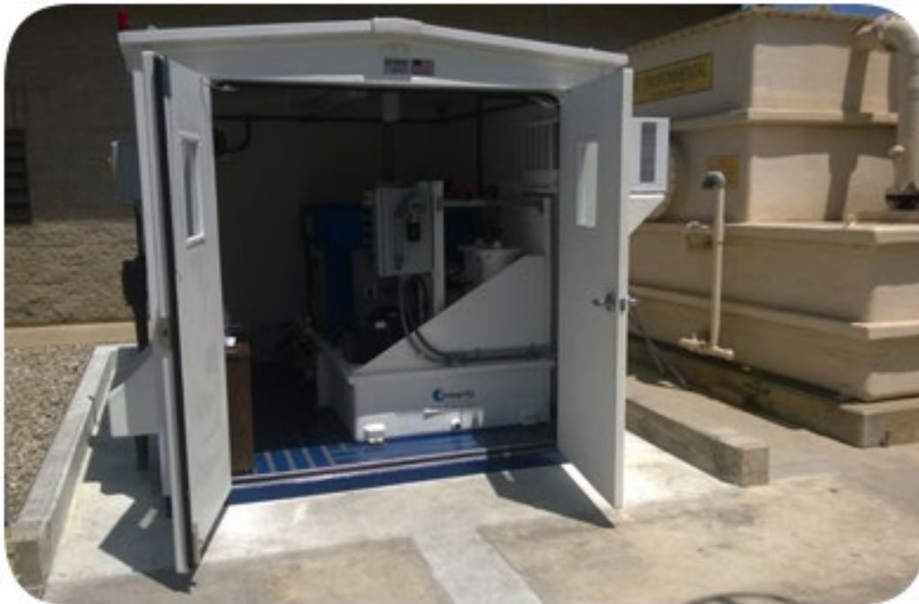
Overall View of Installed Aqueous Ammonia Feed System in an Air Conditioned FRP Enclosure
