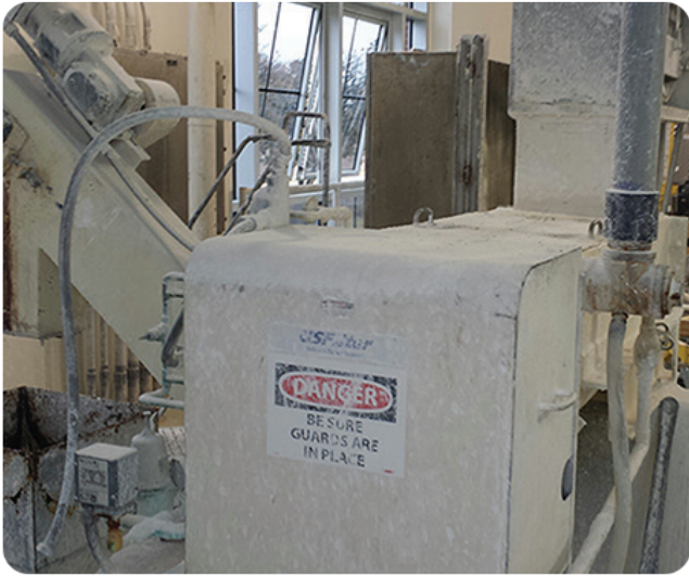
Initial Slaker Condition
