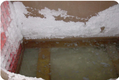
Solids in Sump Up to 29" Thick
