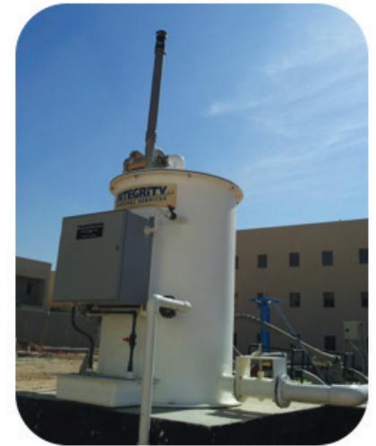
I-BOx™ 42 at Al Bustan Lift Station
