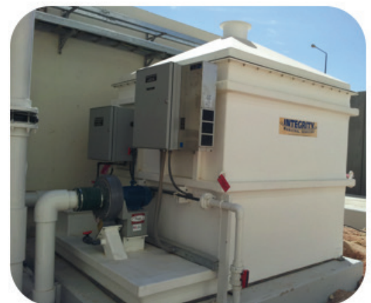
I-BOx™ 7000 at Al Bustan Headworks
