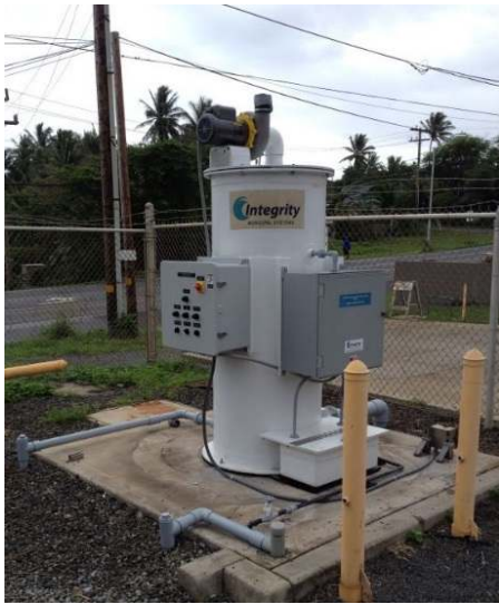
IMS I-BOx® 30 installed at the Hawaiian Homes Wastewater Pump Station.
