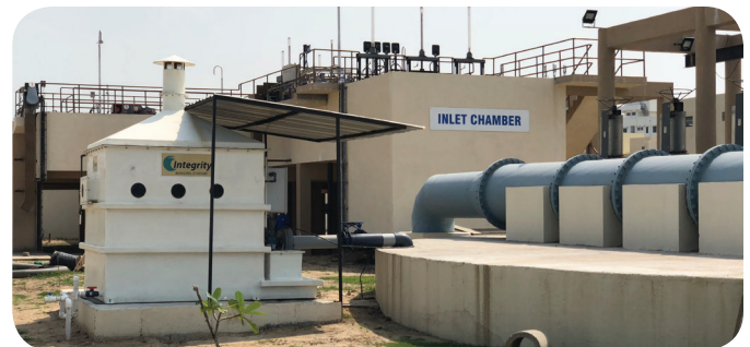
IMS I-BOX® 7000 at Rajivnagar STP
