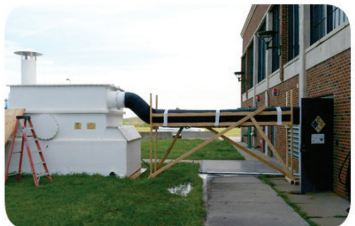
Temporary emergency chlorine scrubber provides protection during rehabilitation
