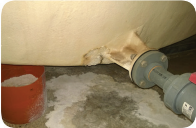
Leak at storage tank drain
