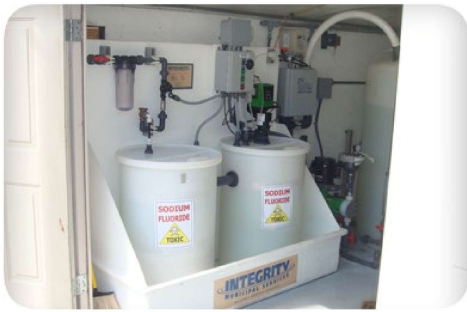
Park Water Company, CA
