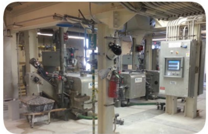
After the new paste-type lime slaker systems were installed, operators can start and stop each system without leaving the control room. Operators and other plant personnel can monitor many aspects of each slaker system from their desk computer. A detailed alarm is reported to the system controls and is displayed on the local screen, complete with history.
