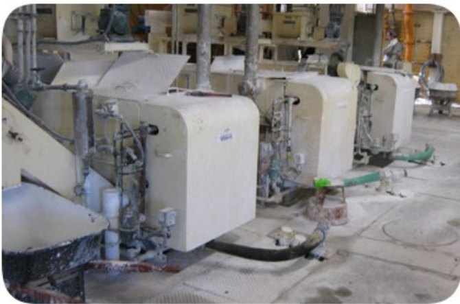
The existing systems consisted of painted carbon steel units which had been severely corroded. The units were in poor condition and required intensive operator intervention.
