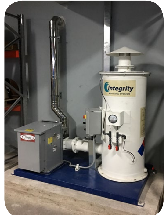
IMS MCS-200 installation at Oil One SA
