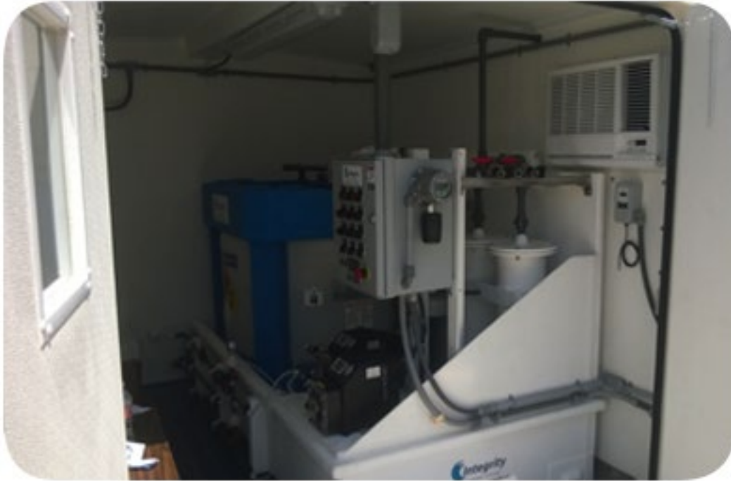
Aqueous Ammonia Feed System Inside Air Conditioned Enclosure
